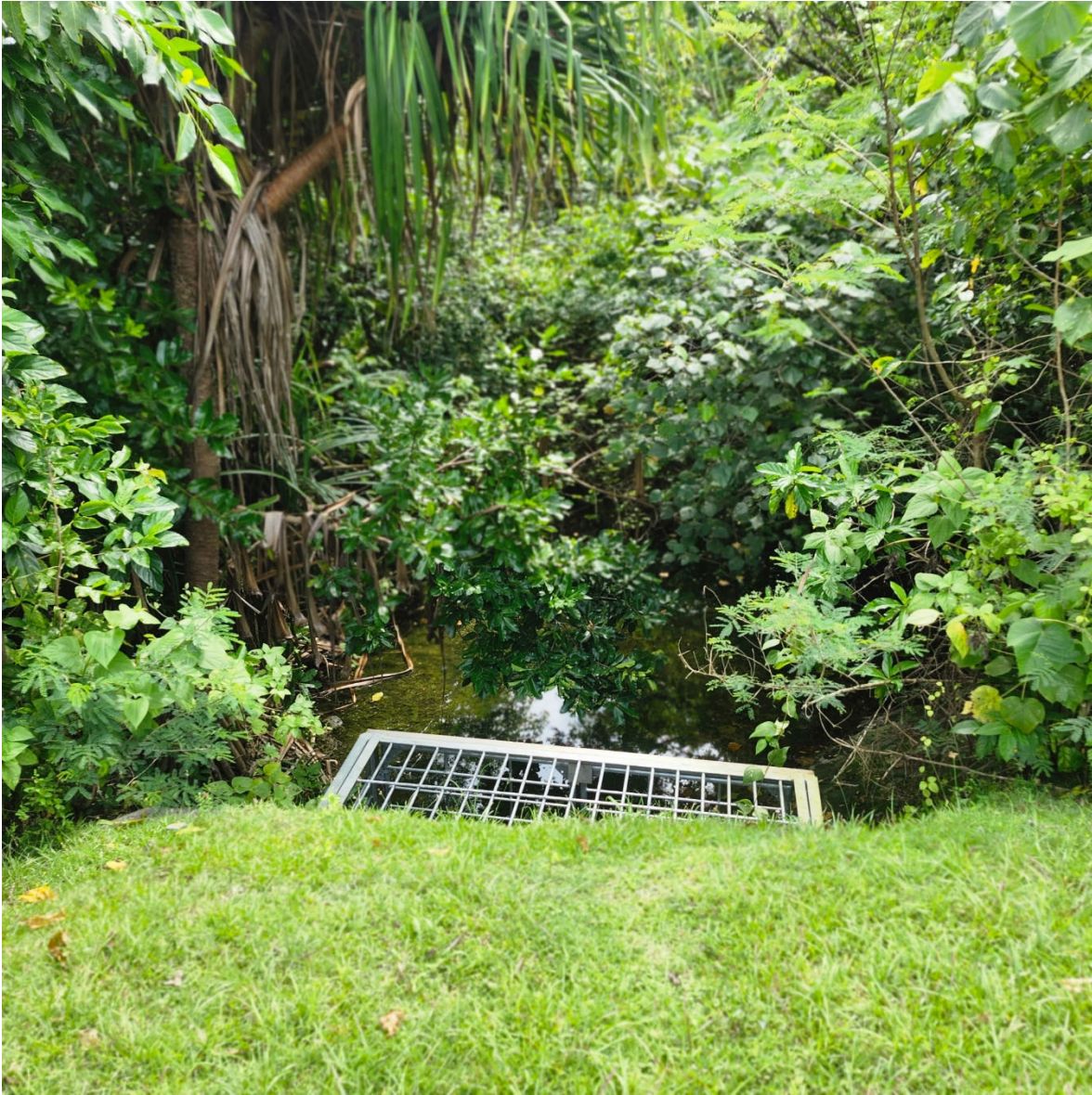
Area 5. Main culvert outlet that feeds the channel leading to priority area 5 wetlands.
