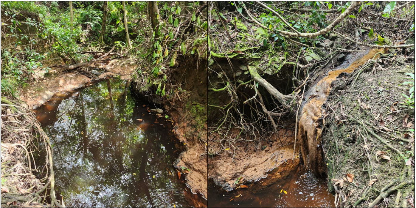
Figure 23. Examples of erosion and stream incision in the vicinity of area 5`, providing opportunities for erosion control and wetland restoration/enhancement.
