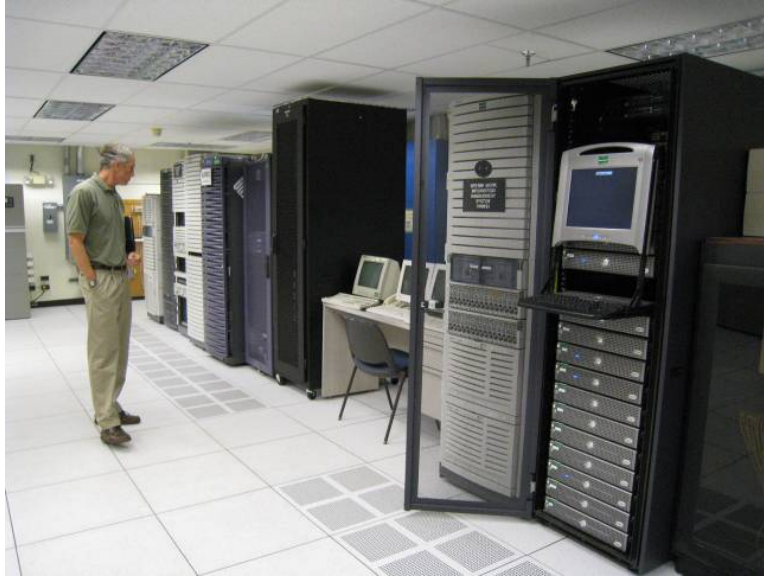
The Defense Enterprise Computing Center Pacific is a test bed for a series of energy efficiency improvements
