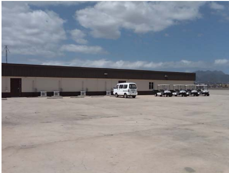
This building at Hickam AFB has spray foam insulation on the roof as part of a demonstration project
